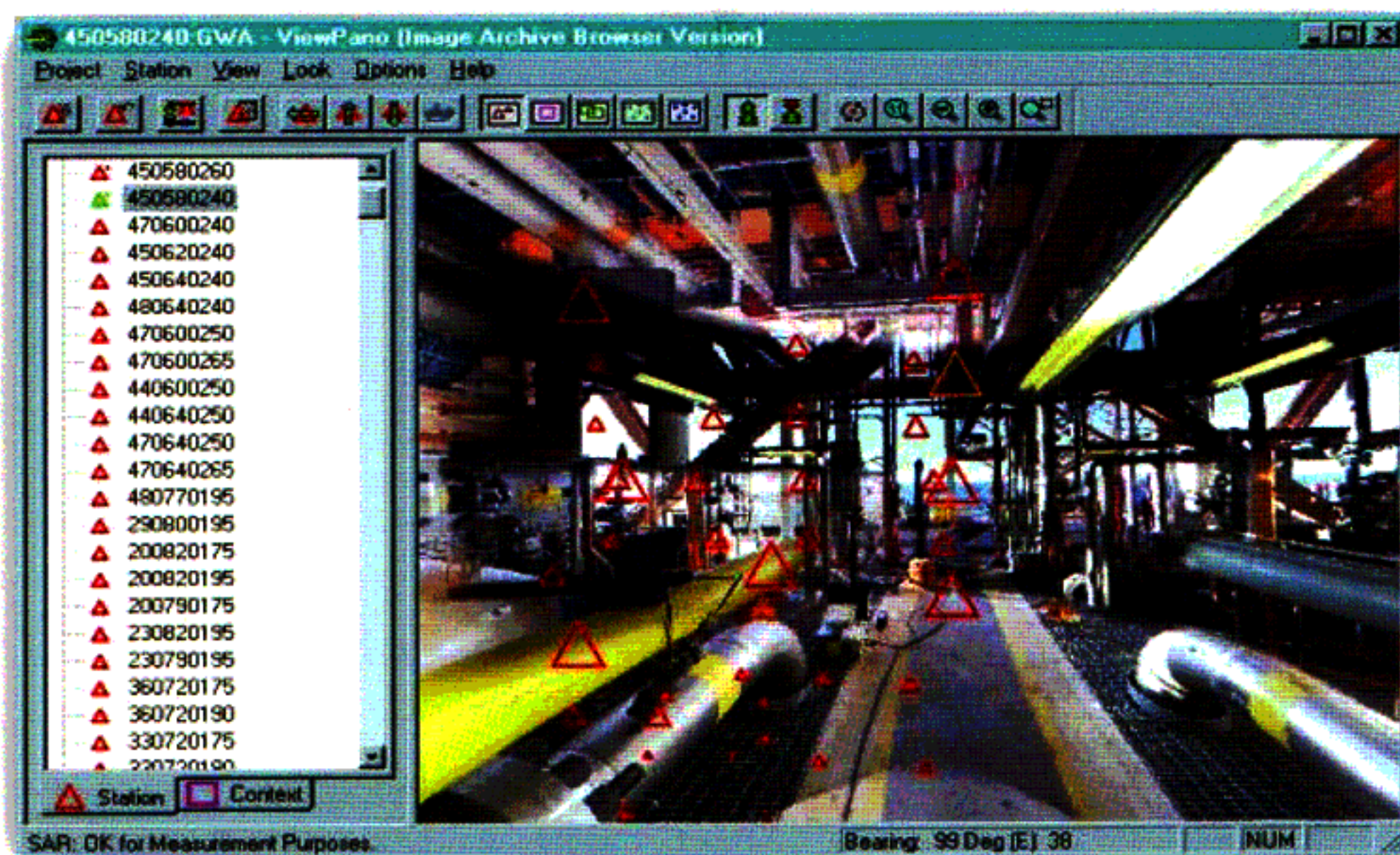
Hazmap Browser depicting Goodwyn A facility. The red triangles are adjacent survey camera stations, smaller ones are further away (some are on the level below the deck shown). (Image courtesy of TWWA)
